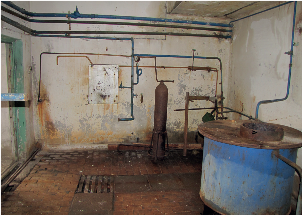
Fig. 2. Dysfunctional chlorination chamber, Sharyngol WWTP
