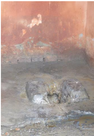
Latrine hole – dangerously big for small children
