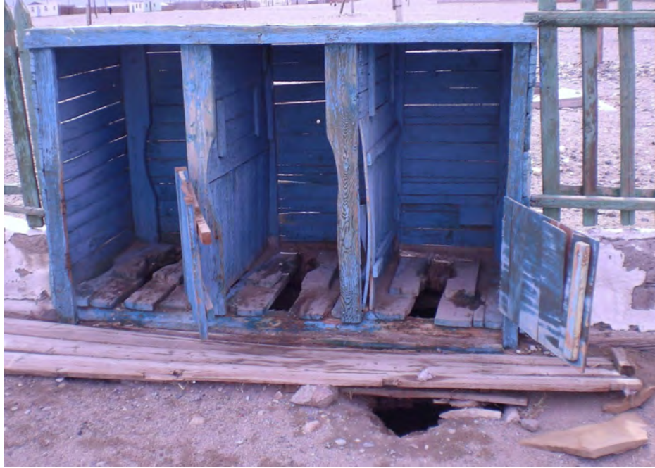
Pit latrine in school. Note the lack of doors and gaping hole in front of one cubicle (photo by Kevin Tayler).
