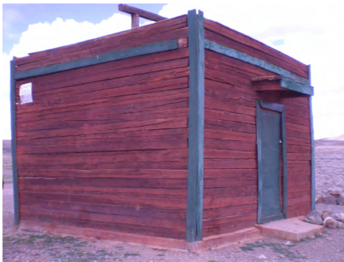
Pump house in Tonkhil Soum, Govi-Altai Aimag. Heating arrangements should be made in the pump house so that the water in the pump riser and supply main never freezes (photo by Kevin Tayler).
