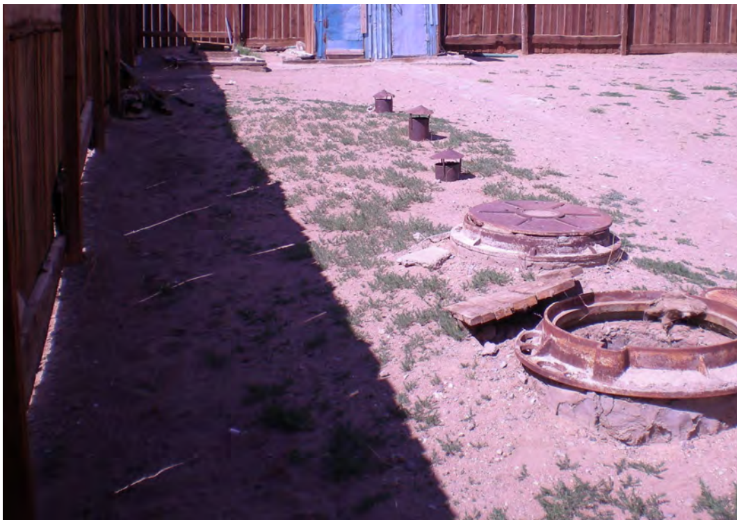
Nonfunctional septic tank. Factors contributing to the failure of the septic tank include freezing of the connecting pipes and lack of water (photo by Kevin Tayler).
